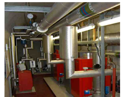
Finished tunnels with new plant equipment.
