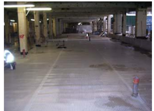
Newton 500 installed to floor.
