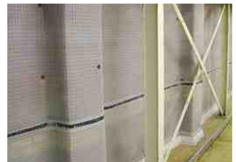
Newton System 500 professionally installed with minimal fixings. Baseboard medium is used to drain water down through the RC slab too the lower level for removal.
