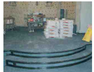
Newton Slimline Flooring installed over damp RC slab.
