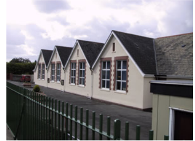
Project Completed - External damp proofing works with top quality finish and achieved within client's budget
