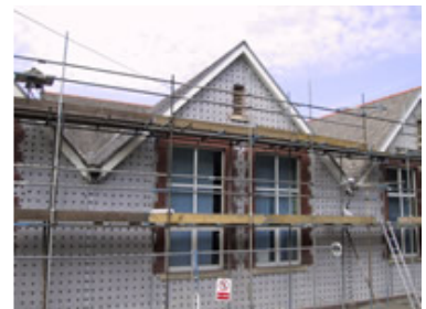
The external application allowed works to be completed without causing disruption to school.
