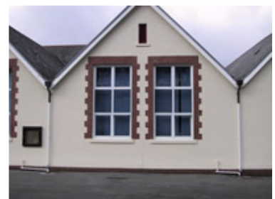
Front view of gable after renders and decorative finishing applied over Newlath 2000 damp proofing membranes
